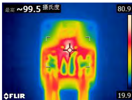
Package Thermography (Input Current 40A)
