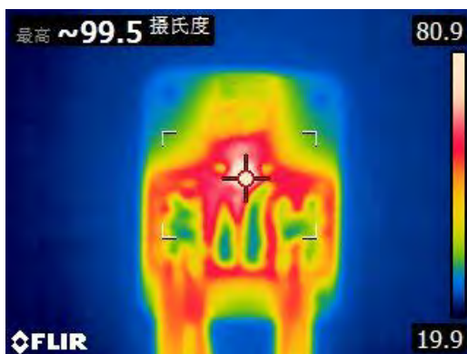
Package Thermography (Input Current 40A)
